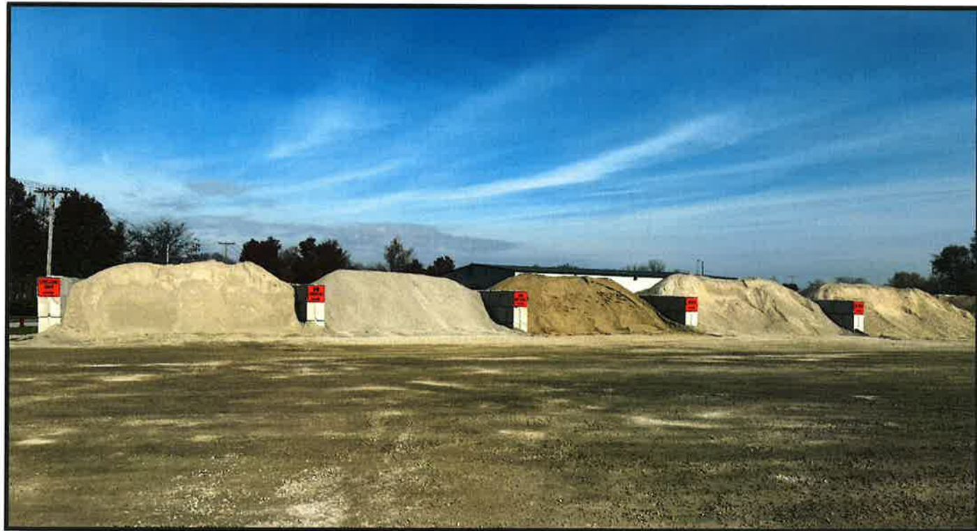
Picture 3: Example: Aggregate (Stone and Sand) Storage Bunkers
